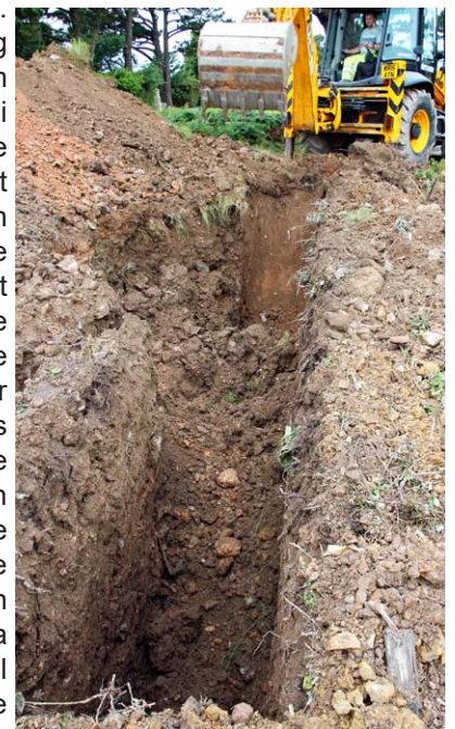
A three metre deep trench that has just collapsed.
